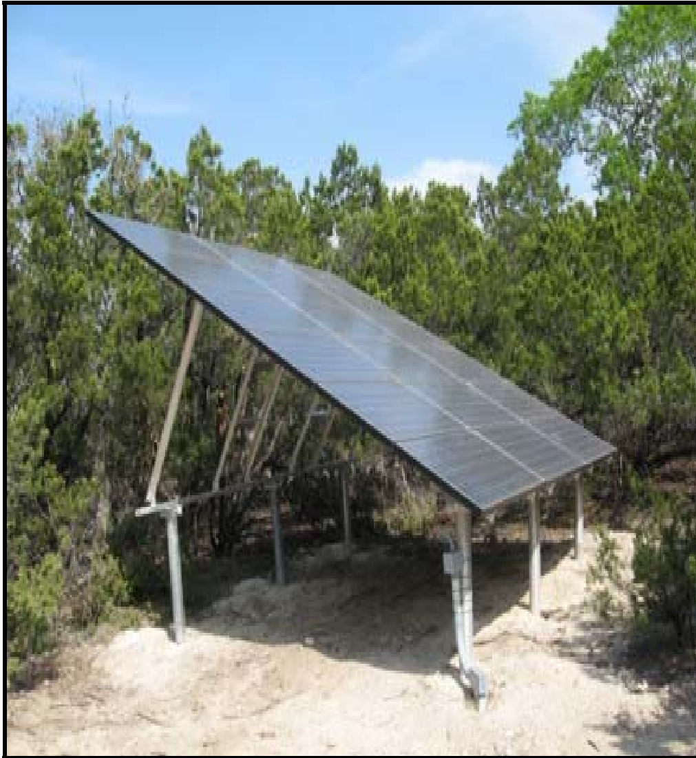
Elevated Ground Mount
